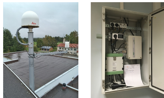
Figure 5. Typical installation of most ESTPOS stations – an AR25 Choke Ring radome antenna with the Vaisala WXT520 meteo sensor and an equipment housing containing a GR25 receiver and a converter for the meteo sensor
