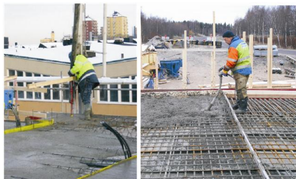
Fig. 7. Self-Compacting Concrete Casting (photo on the left) with no need to use a compacting vibrator (as seen on photo on the right)
