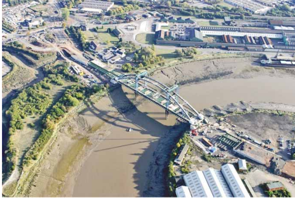
Fig. 2. NSDR PFI road project and River Usk Bridge under construction (Courtesy: MorganEST Rugby Office Archive)
